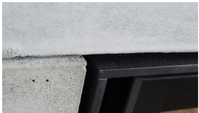
Illustration 3: Detailed view: Gap between the mounting frame and thermal concrete cladding
